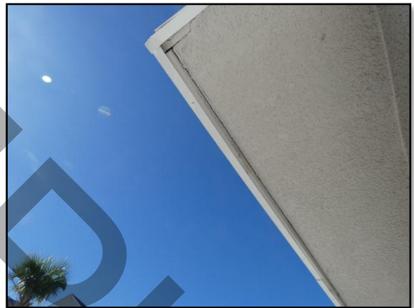
18 - Missing drainage accessory at horizontal / vertical transition. M08_(2388)
