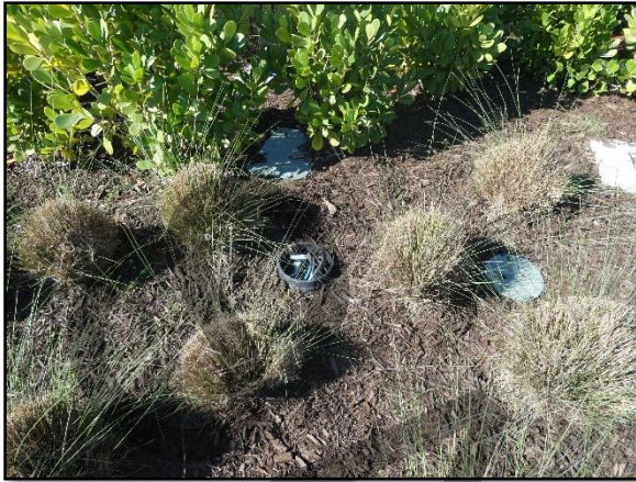
80 – Missing valve box / utility vault cover(s). M08_(2295)
