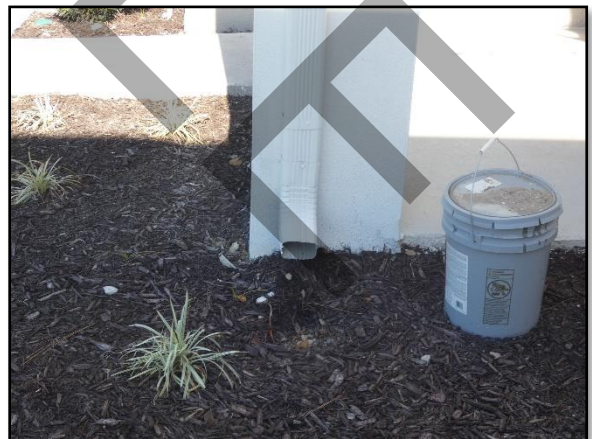
75 - Improper discharge of gutter downspout. M08_(2545)
