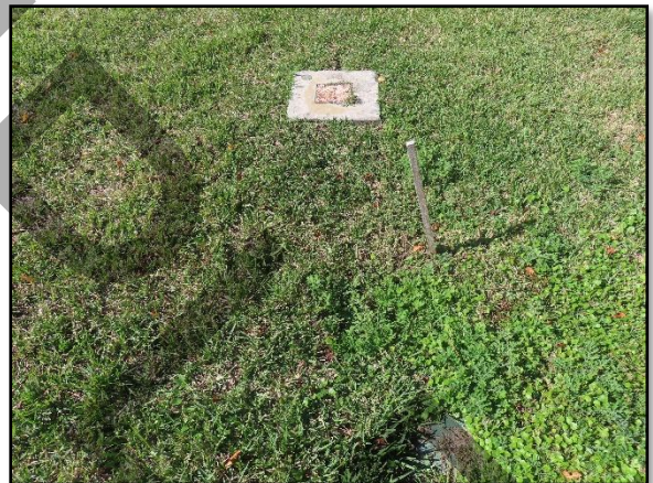
69 - Obstructed / debris at stormwater drain. M19_(1066)
