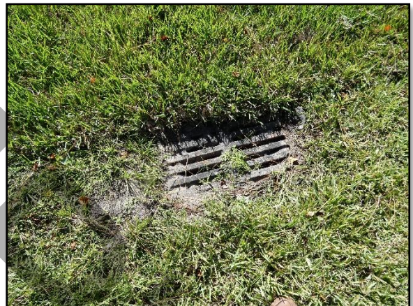
73 - Obstructed / debris at stormwater drain. M57_(1166)
