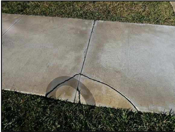
60 - Cracked / damaged sidewalk. M57_(147)
