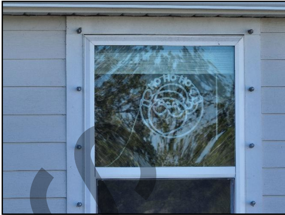
33 - Missing / deteriorated sealant. M19_UAV(1347)
