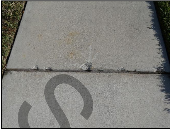
54 - Cracked / damaged sidewalk. M57_(124)
