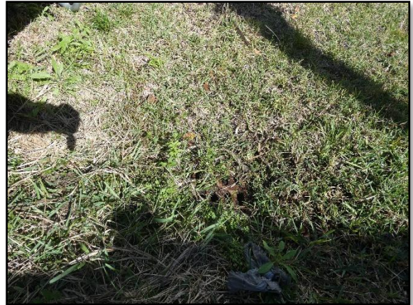
67 - Obstructed / debris at stormwater drain. M08_(2394)
