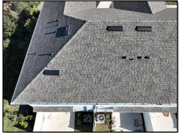
2 - Missing / slipped shingle(s). M19_UAV(1474)
