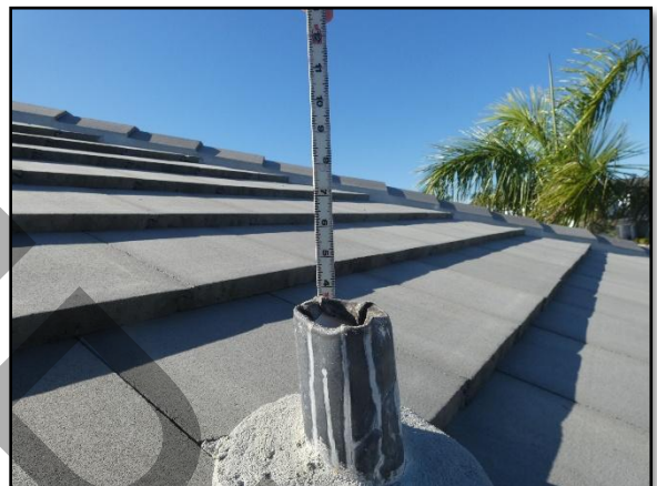
10 - Vent height less than 6" above roof deck. M08_(2230)
