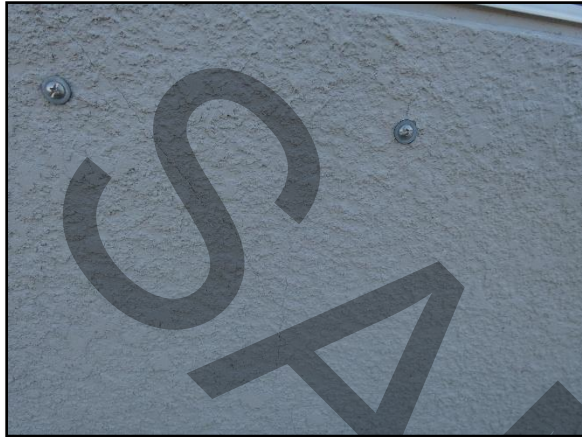
11 - Stucco cracks. M08_(2376)
