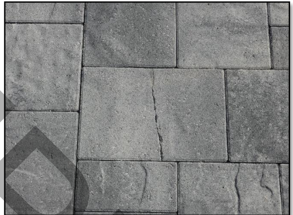
63 - Damaged / missing pavers. M08_(2235)
