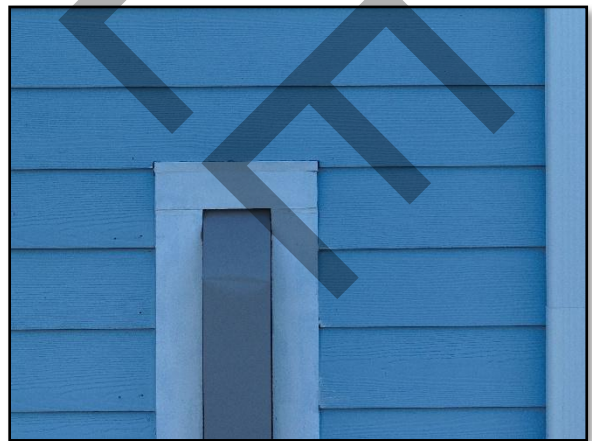
20 - Improper clearance at Z-flashing. M19_UAV(1252)
