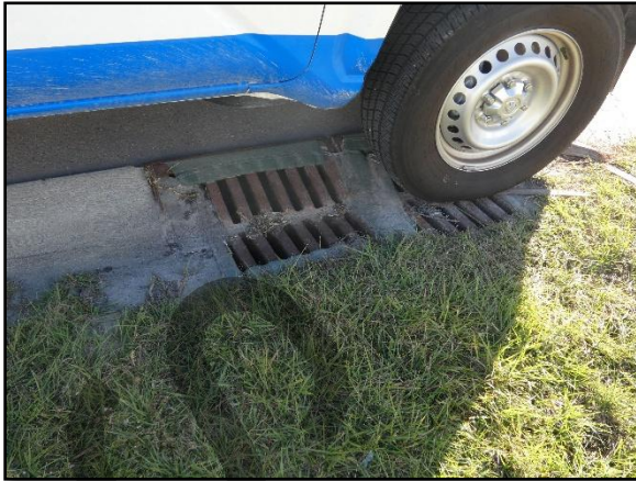
76 - Damaged / missing filter fabric. M57_(165)
