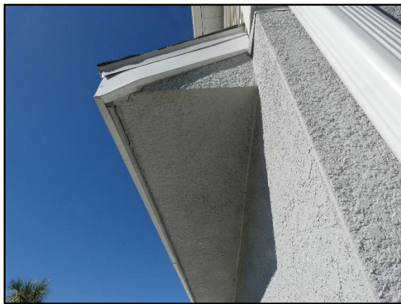
19 - Missing drainage accessory at horizontal / vertical transition. M08_(2454)
