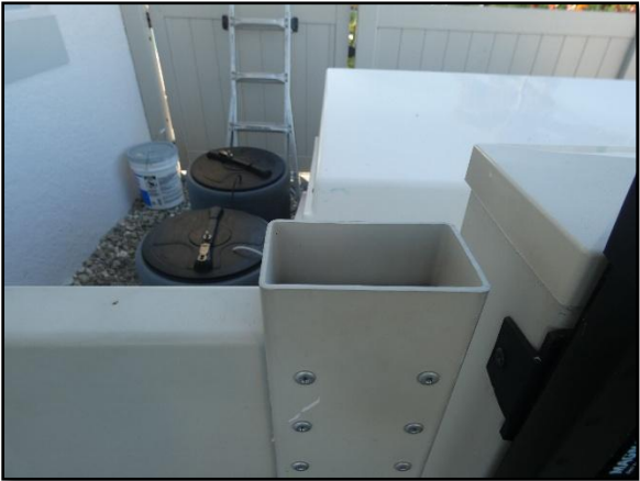
99 - Missing caps on fence post(s). M08_(2065)
