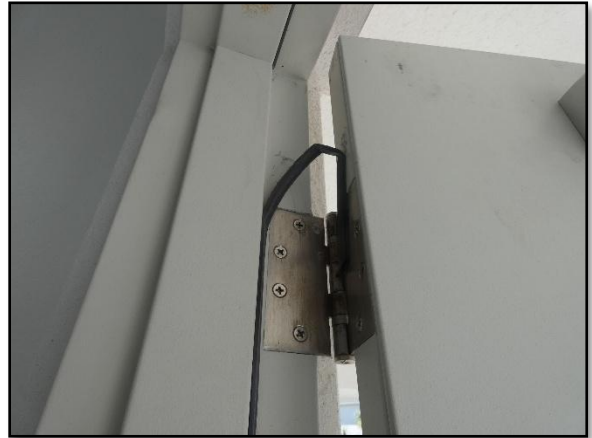
28 - Damaged weatherstripping. M08_(2121)
