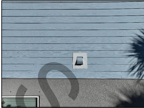
21 - Improper clearance at Z-flashing. M19_UAV(1267)
