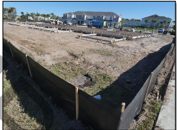
79 - Damaged / missing filter fabric. M08_(2315)
