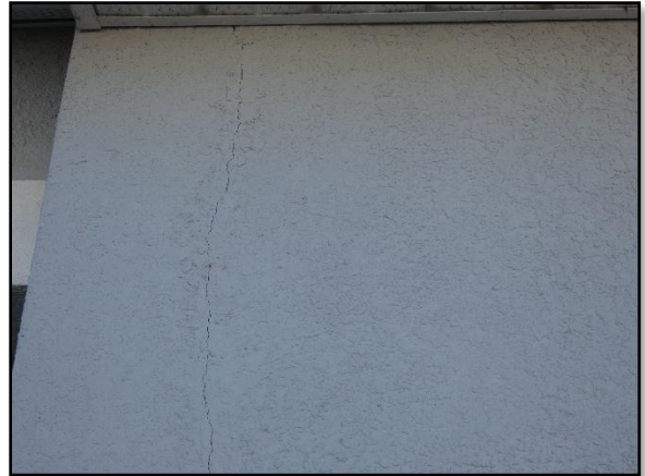
12 - Stucco cracks. M08_(2418)
