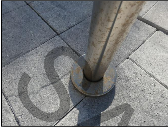
40 - Corroded escutcheon at handrail / ladder. M08_(2007)
