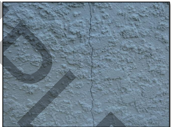
14 - Stucco cracks. M57_(427)
