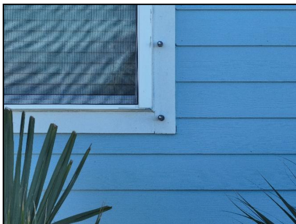
25 - Missing sealant at siding joints. M19_UAV(1238)
