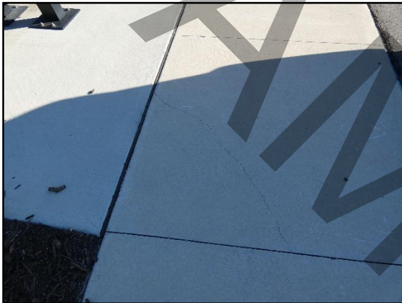
56 - Cracked / damaged sidewalk. M57_(128)
