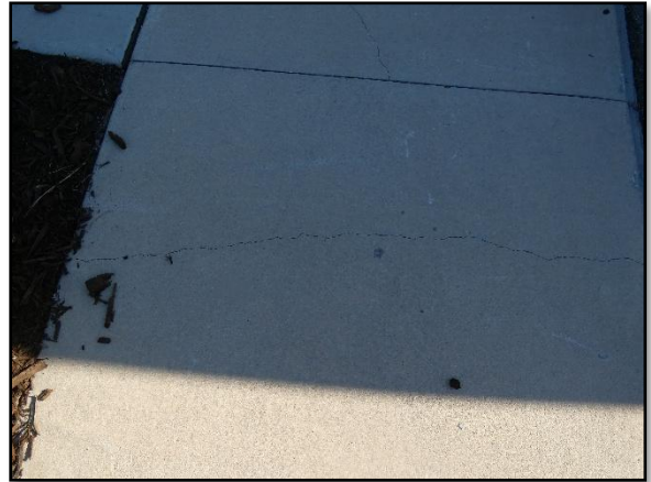
55 - Cracked / damaged sidewalk. M57_(127)
