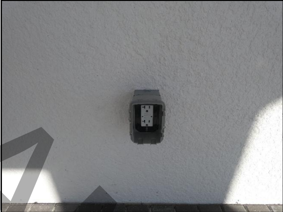
39 - Missing weatherproof electrical cover. M08_(2084)
