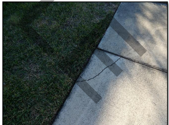
59 - Cracked / damaged sidewalk. M57_(142)
