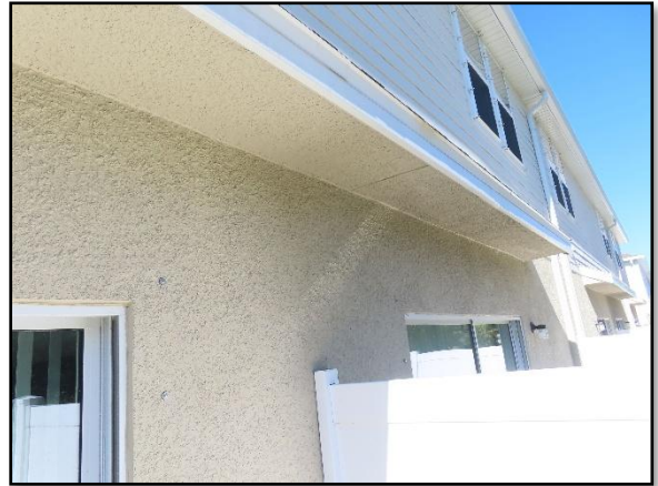
16 - Missing drainage accessory at horizontal / vertical transition. M19_(1032)
