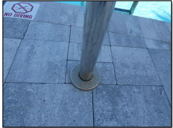
41 - Corroded escutcheon at handrail / ladder. M08_(2030)
