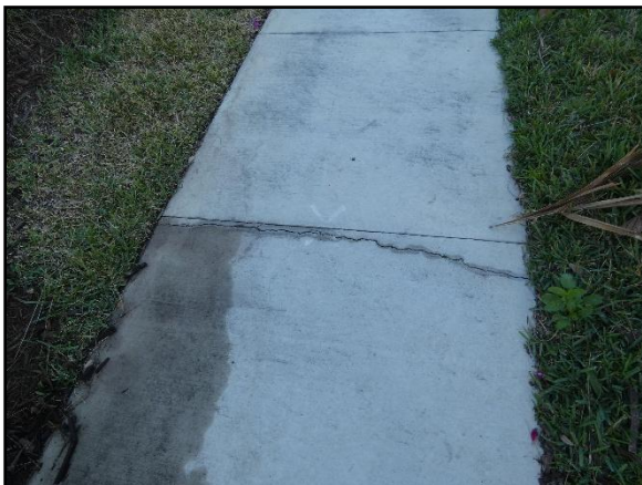
58 - Cracked / damaged sidewalk. M57_(133)
