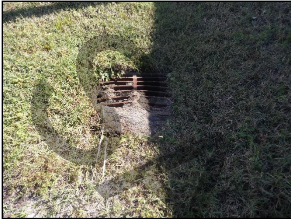
66 - Obstructed / debris at stormwater drain. M08_(2352)
