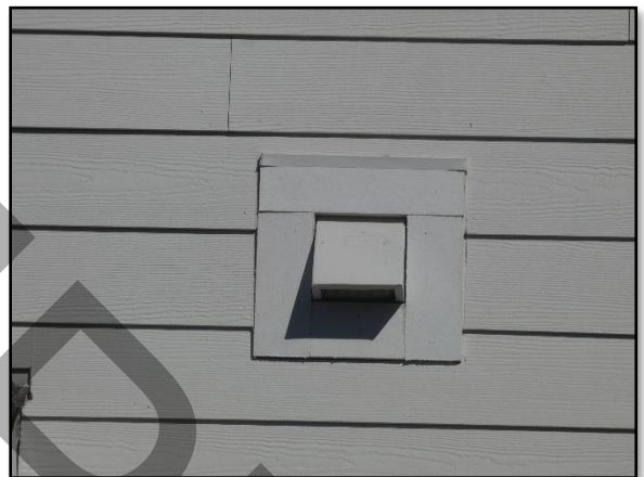
24 - Improper clearance at Z-flashing. M08_(2396)
