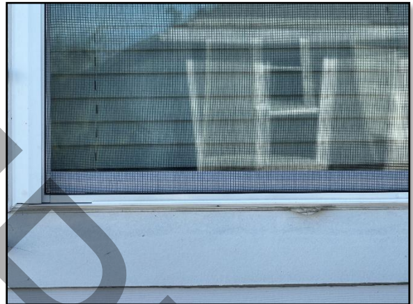
30 - Missing / deteriorated sealant. M19_UAV(1295)
