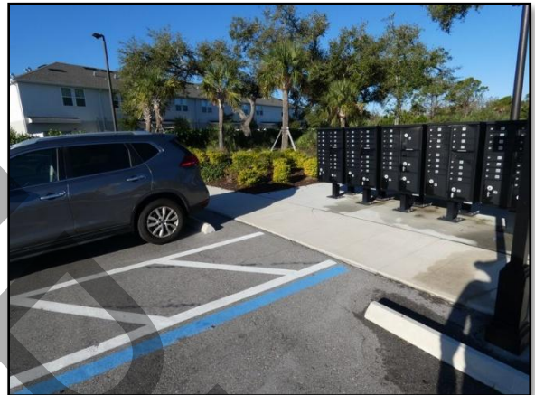
51 - Missing detectable warning. M57_(140)
