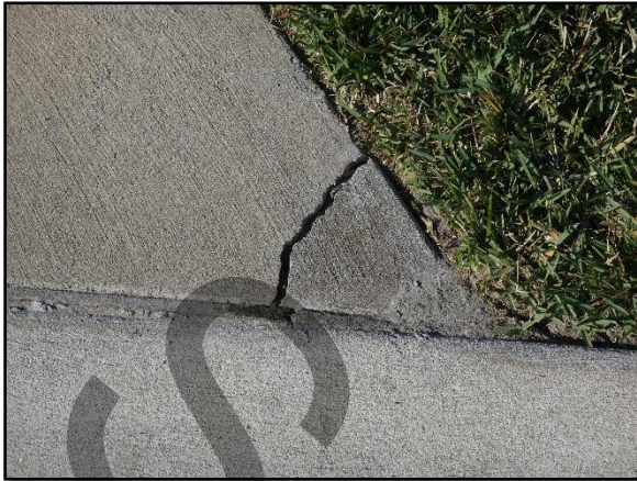
48 - Damaged driveway corner. M57_(163)
