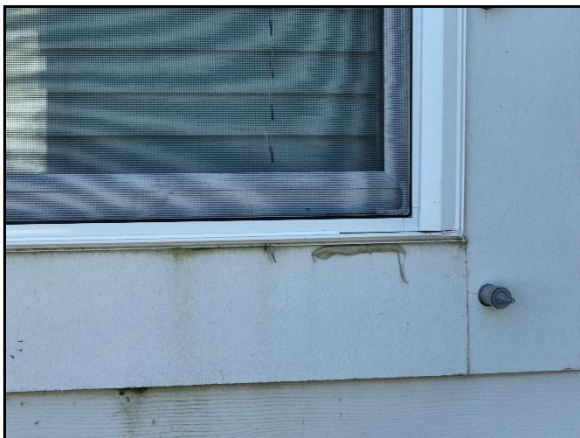
31 - Missing / deteriorated sealant. M19_UAV(1424)
