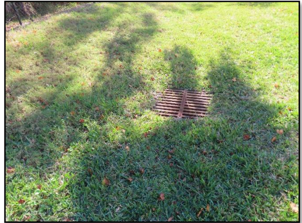
71 - Obstructed / debris at stormwater drain. M19_(1023)
