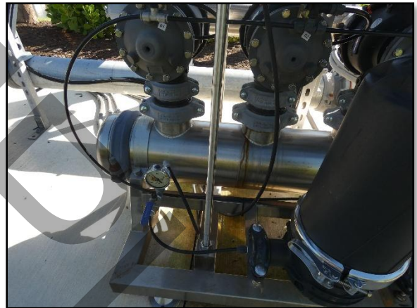
83 – Evidence of leak. M08_(2261)
