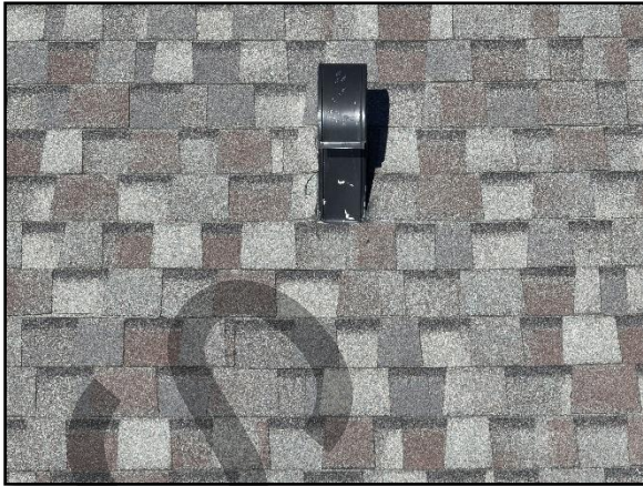
7 - Shingles over downside flange(s). M19_UAV(1373)
