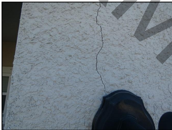
13 - Stucco cracks. M57_(351)
