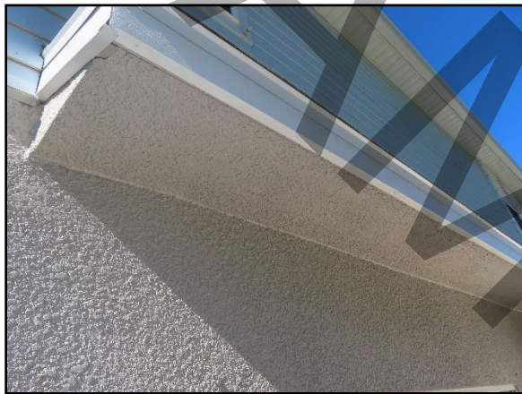
17 - Missing drainage accessory at horizontal / vertical transition. M19_(1078)
