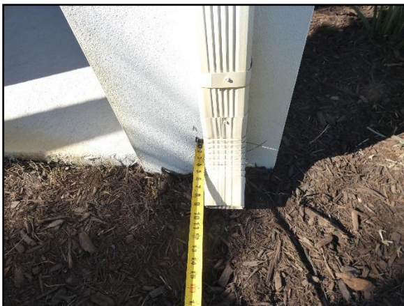
74 - Improper discharge of gutter downspout. M08_(2527)
