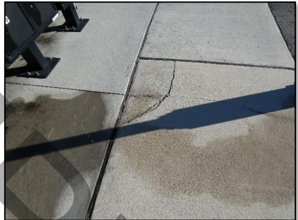
57 - Cracked / damaged sidewalk. M57_(130)
