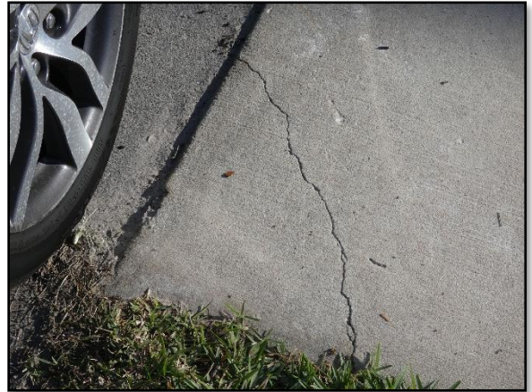
61 - Cracked / damaged sidewalk. M57_(170)
