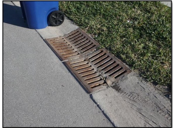
77 - Damaged / missing filter fabric. M57_(167)
