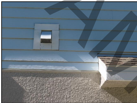
23 - Improper clearance at Z-flashing. M19_(1076)
