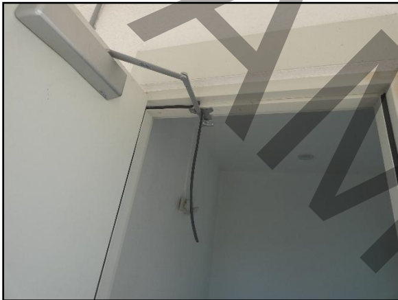
29 - Damaged weatherstripping. M08_(2135)
