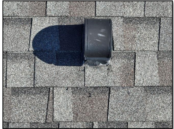
8 - Shingles over downside flange(s). M19_UAV(1508)
