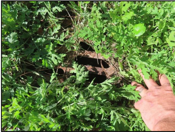
70 - Obstructed / debris at stormwater drain. M19_(1067)
