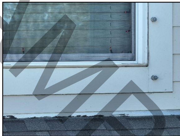
35 - Missing / deteriorated sealant. M19_UAV(1410)
