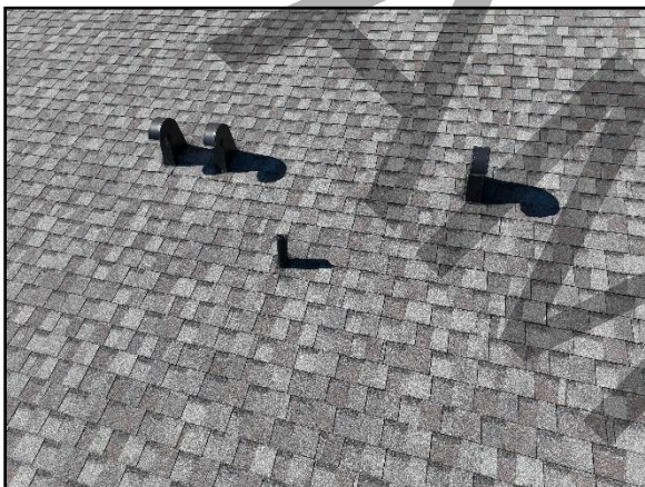
9 - Shingles over downside flange(s). M19_UAV(1620)
