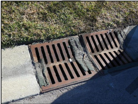
78 - Damaged / missing filter fabric. M57_(188)
