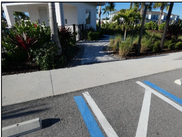
52 - Missing detectable warning. M57_(190)
