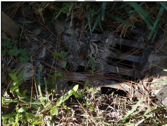
72 - Obstructed / debris at stormwater drain. M57_(1154)
