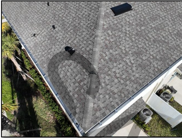
1 - Missing / slipped shingle(s). M19_UAV(1393)
