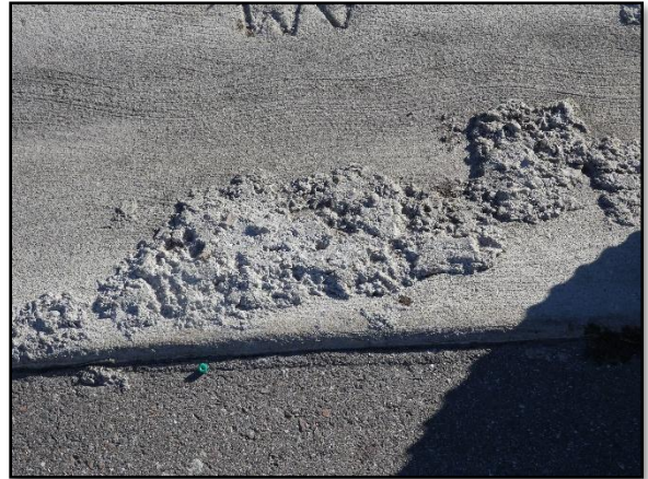
49 - Concrete spoil in gutter. M57_(154)
