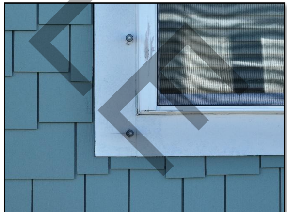
32 - Missing / deteriorated sealant. M19_UAV(1296)
