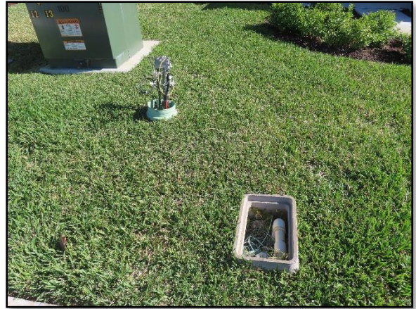
81 – Missing valve box / utility vault cover(s). M19_(1094)
