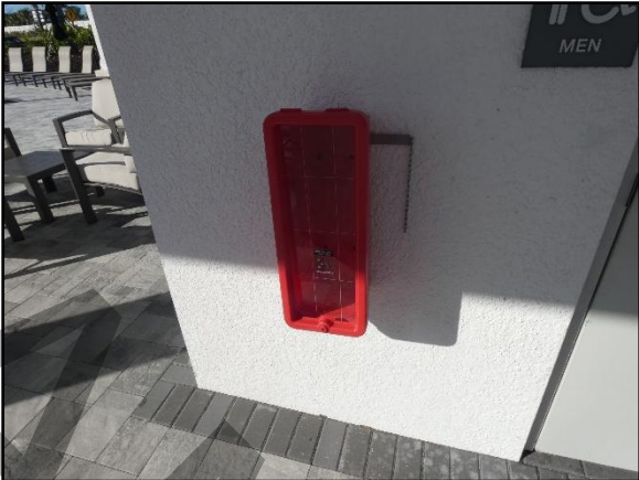
36 - Missing fire extinguisher. M08_(2093)
