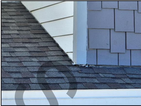
27 - Missing sealant at siding joints. M19_UAV(1645)
