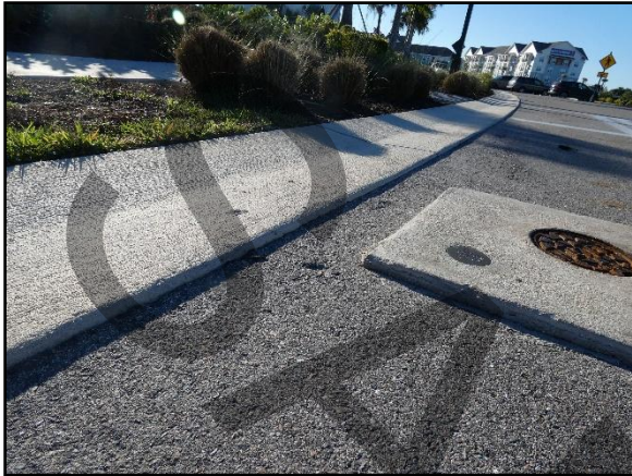
44 - Final lift not completed. M57_(103)
