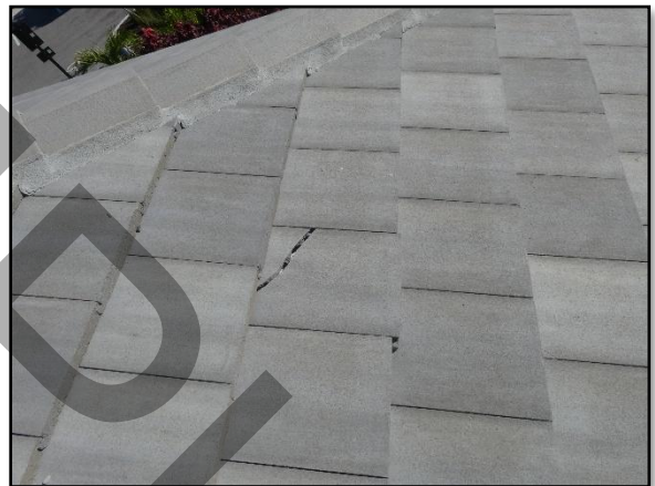
4 - Broken tile(s). M08_(2213)
