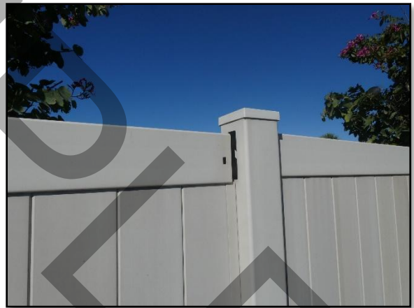
97 - Loose / disconnected / missing fencing section. M08_(2323)
