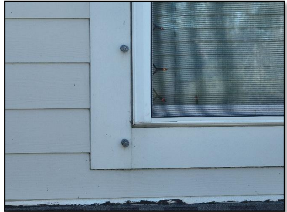
34 - Missing / deteriorated sealant. M19_UAV(1409)
