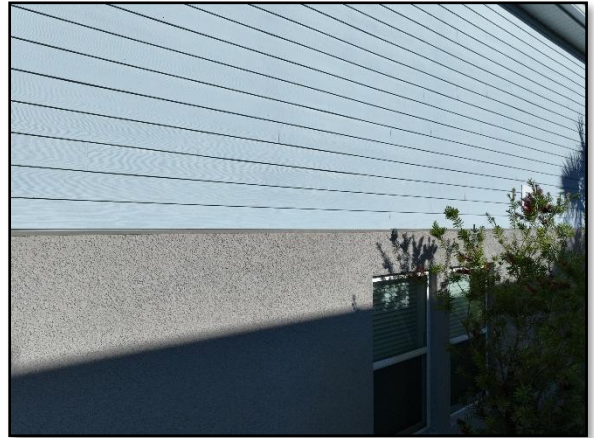
22 - Improper clearance at Z-flashing. M19_UAV(1265)
