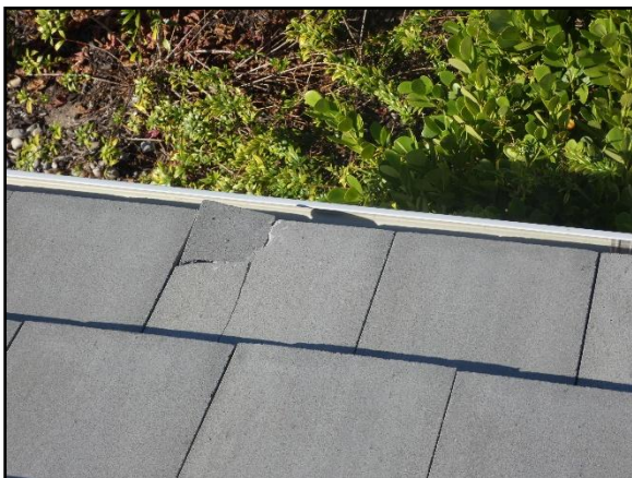
5 - Broken tile(s). M08_(2218)
