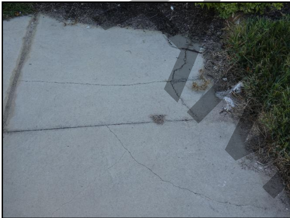
62 - Cracked / damaged sidewalk. M57_(172)
