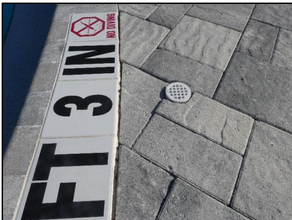
64 - Uneven / sunken / displaced pavers. M08_(2035)
