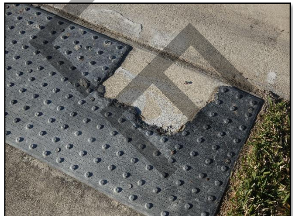
53 - Damaged detectable warnings. M57_(159)
