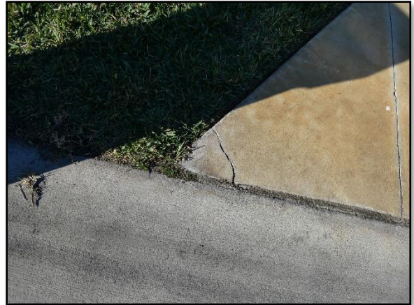
45 - Damaged driveway corner. M57_(148)
